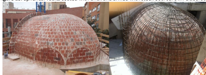
Figure 13. Spherical vaults coated with brick and armed with steel. Source: own elaboration
