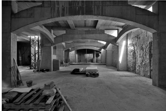
Figure 4. Current status of works in the basement of the Romanian Orthodox Church in Barcelona. [ http://www.bisericabarcelona.es/ ]. Source: own elaboration
