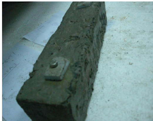
Figure 8. The desquamation of concrete surface owing to freezing-thawing cycles. Source: Own elaboration.
