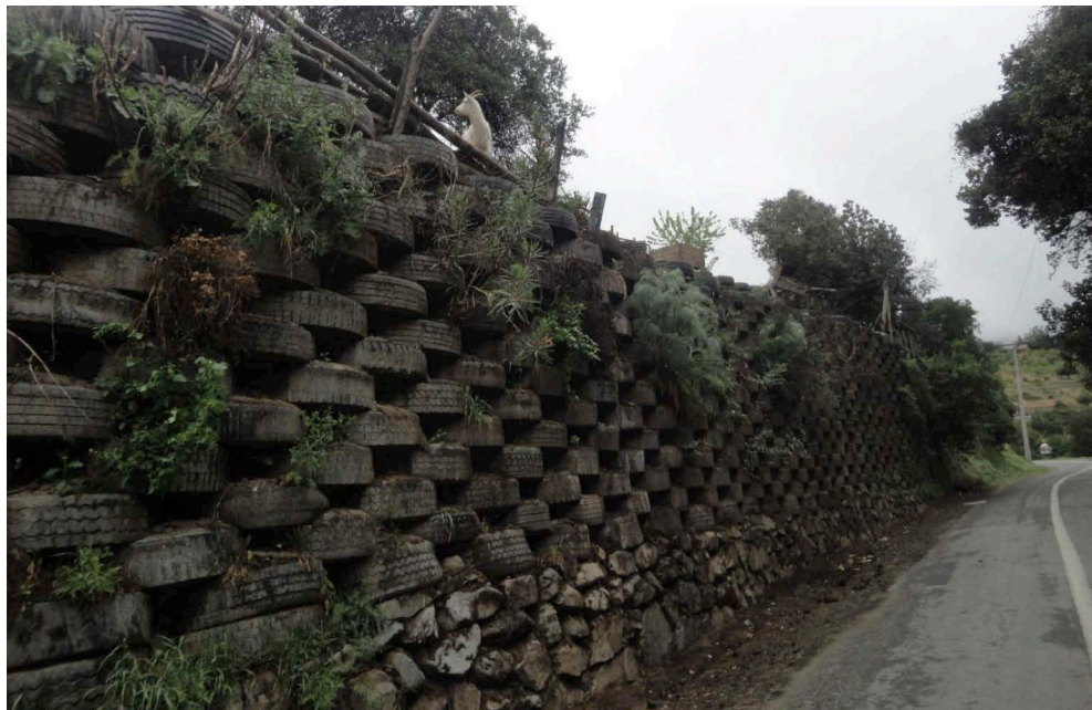
Figure 5. Retaining wall in the La Vega sector, Olmué. (Photography: courtesy of Tania Estay)
