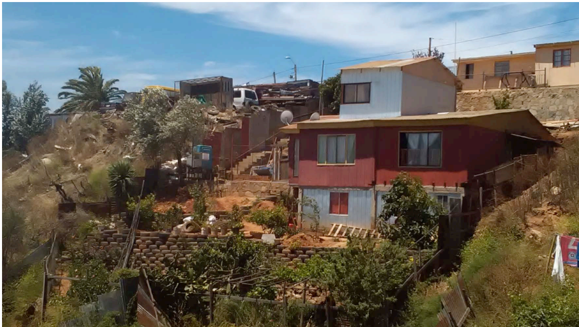
Figure 4. Retaining wall in Cerro Las Cañas, Valparaíso. (Photo courtesy of Claudio Peña)
