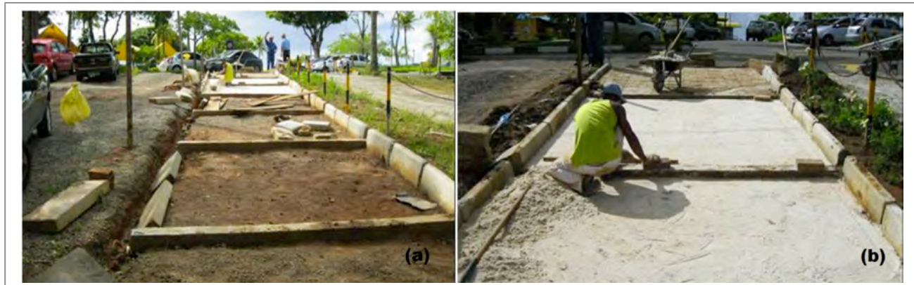
Figure 6. a) Installation of the edge courses and transversal beams; b) Settling of the blocks in the sand layer
