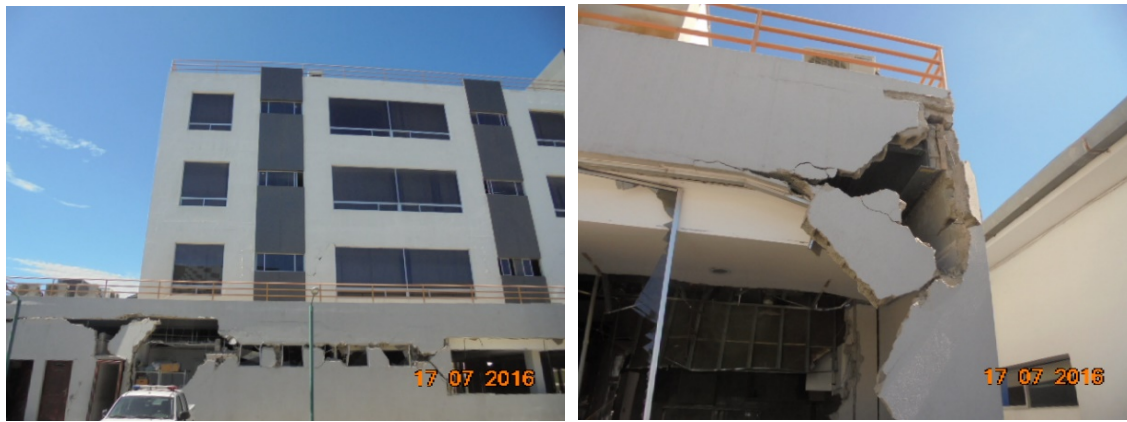
Figure 1. The staff’s residential building of the Manta UVC is a 4-floor steel structure, with cantilevers in the floor plan only, whose masonry was largely damaged. Source: (Aguiar et al., 2016)
