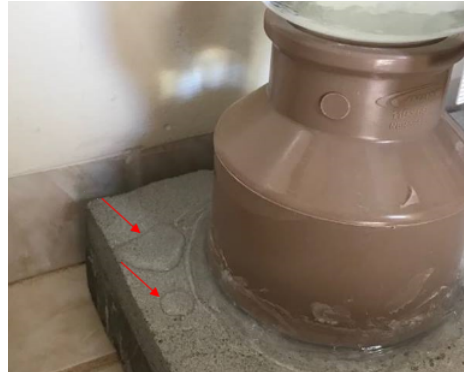
Figure 11. Water surfaced on the surface of the mortar coating
