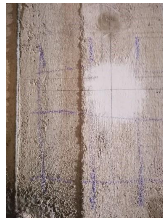
Figure 2. Area of column selected for measurement with rebar location marked with crayon
